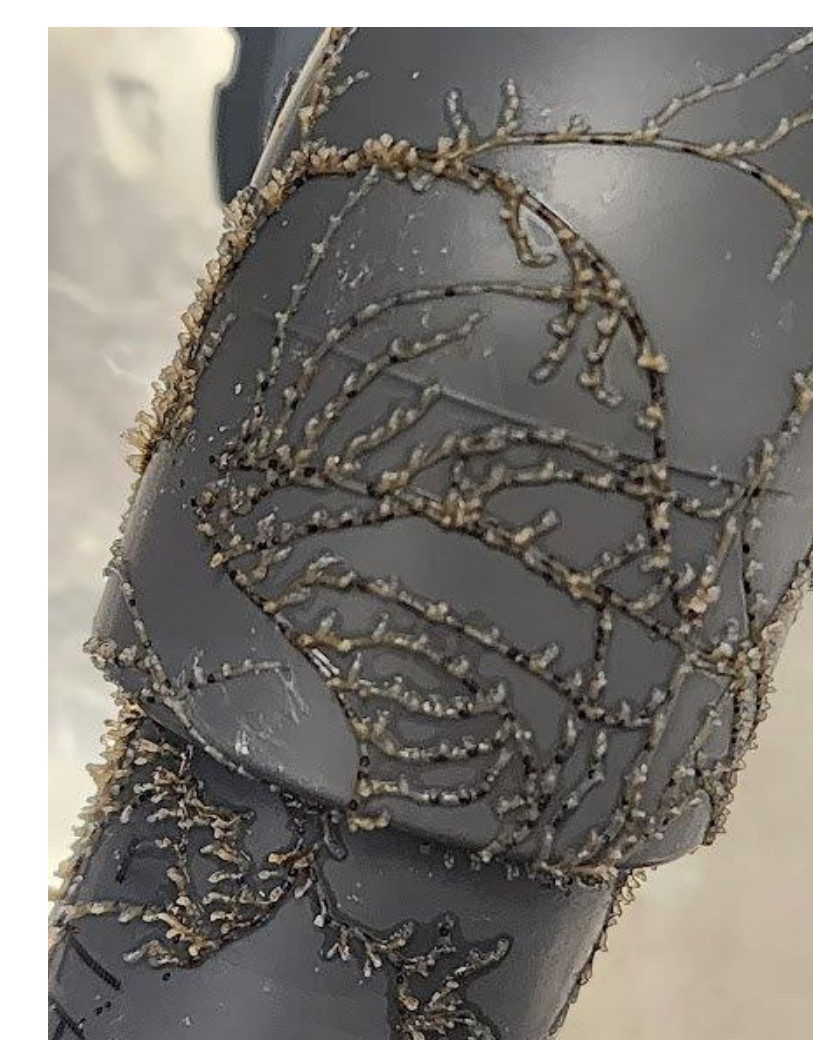
Figure 11: Bryozoan colony clinging to a pipe inside of the sump.
